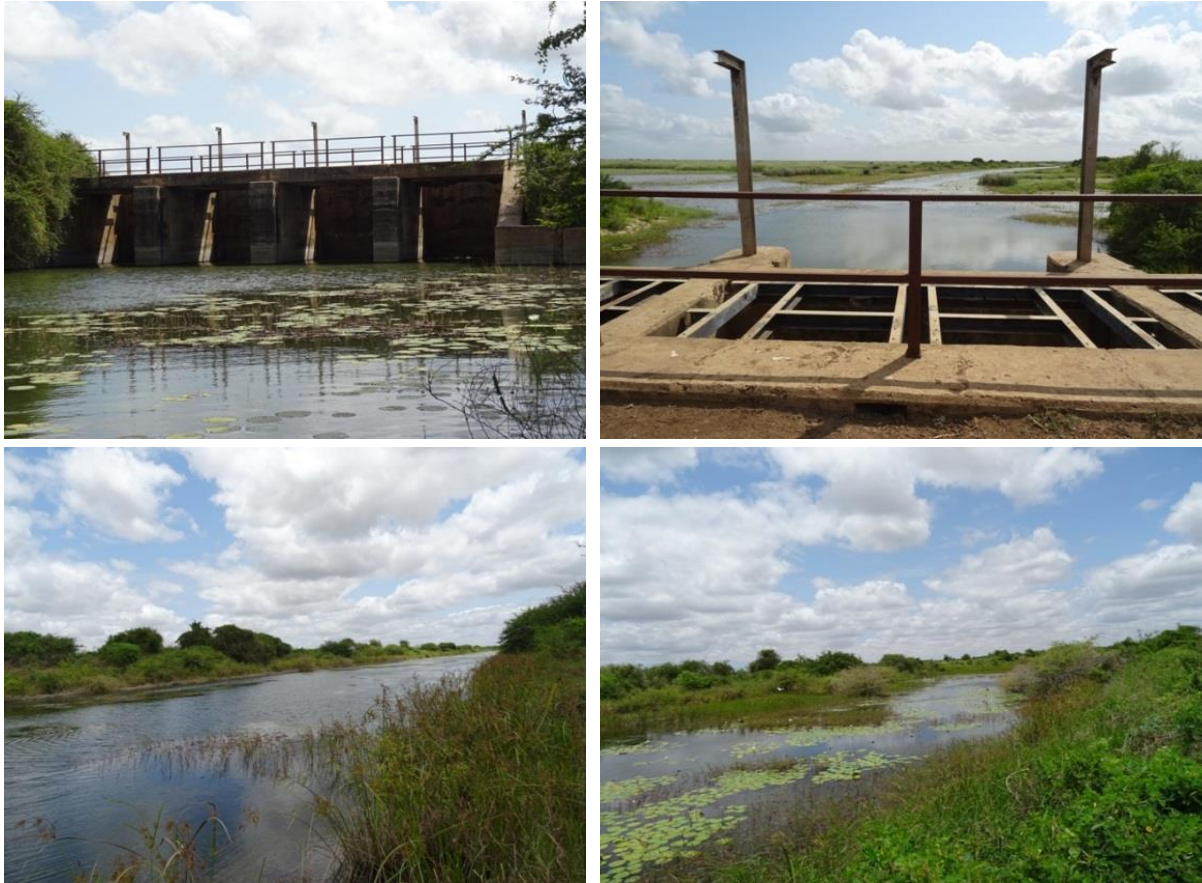
Figure 3-10 Photo shows outlet canal and head regulator
