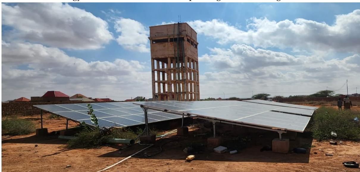
Figure 3-10: Solar Panels for supply of power for Borehole for Durdur Water co. Ltd
