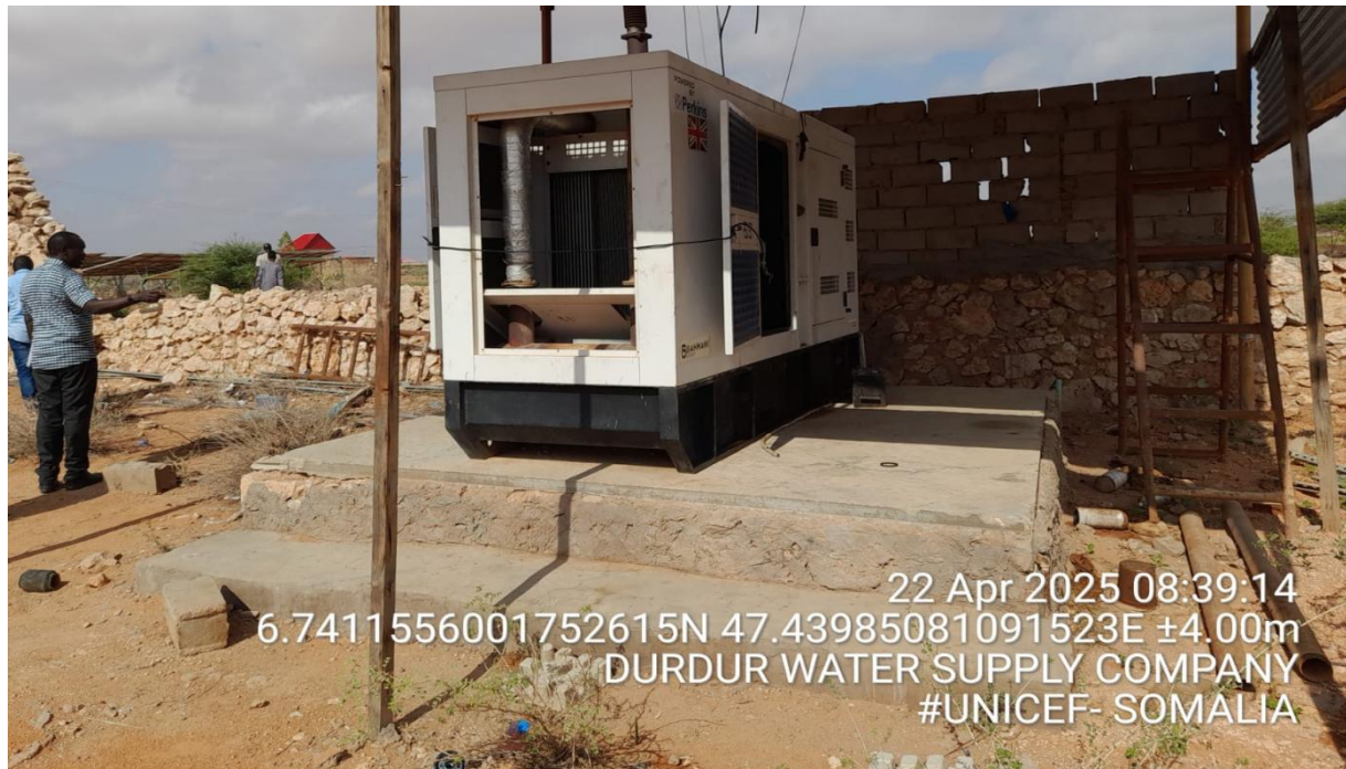
Figure 3-11: Generator for supply of power for Borehole for Durdur Water Supply
