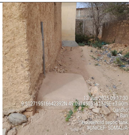
Figure 3.12: Typical Household Septic Tank within the urban areas of Qardho town
