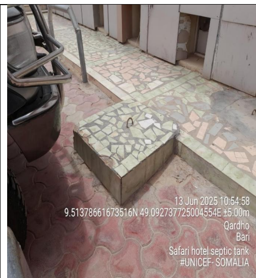
Figure 3.13: Properly lined Septic tank for Safari Hotel in Qardho town
